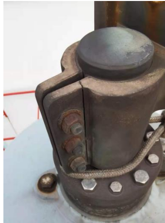
Fig.1 H59 brass alloy terminals with crack
